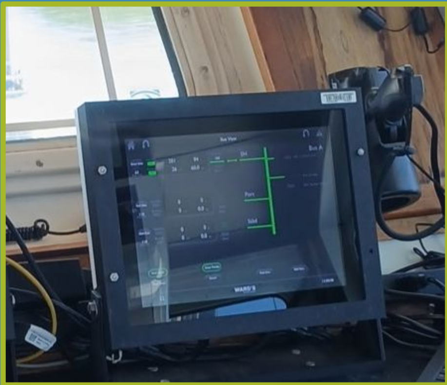
Wheelhouse Switchboard Monitoring/control in Bridge
