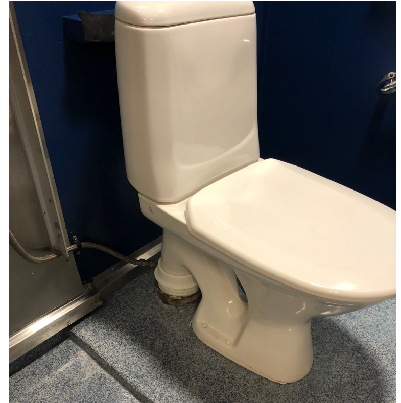
New installed heads on R/V Langseth sourced in Europe due to the flange and piping size.
