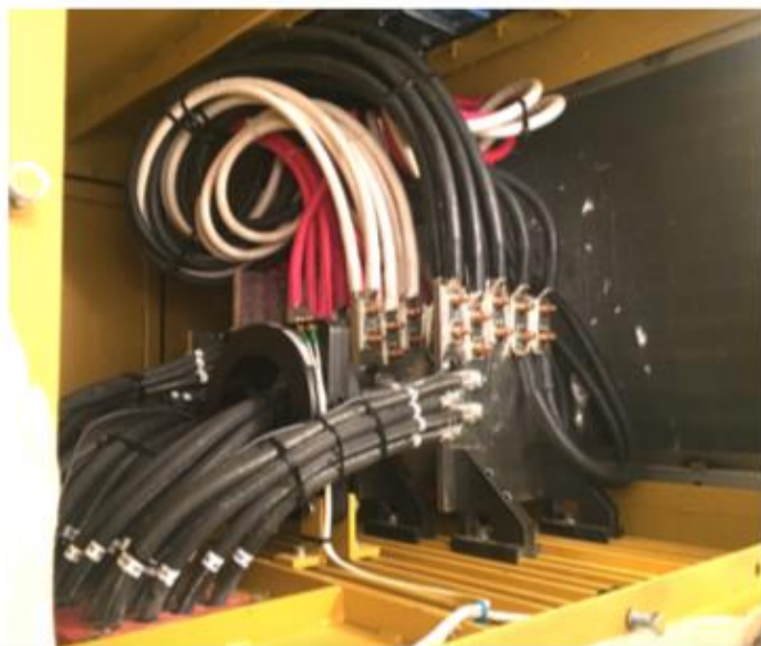
Cable connections in new generator
