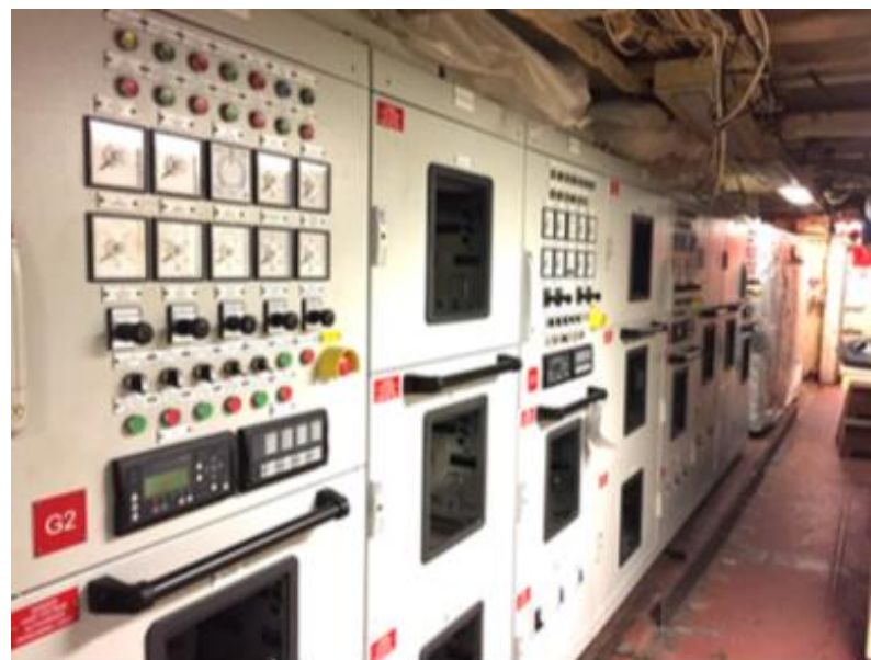
New Switchboards in place
