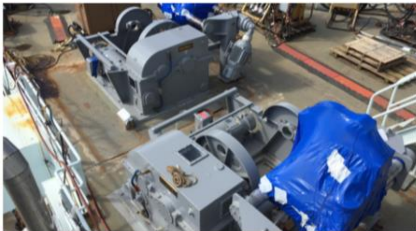
Refurbished hydro-winsches in place
