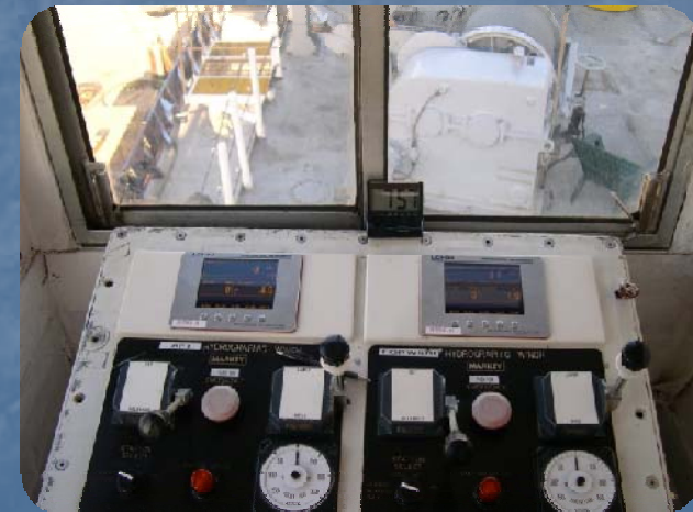
Revelle Hydro Control Station
