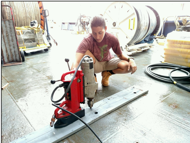
Martine Holmquist working with a magnetic drill to make holes into 1" steel to bolt a winch onto the deck of the R/V Marcus G. Langseth . Photo by Kate Tremblay.
