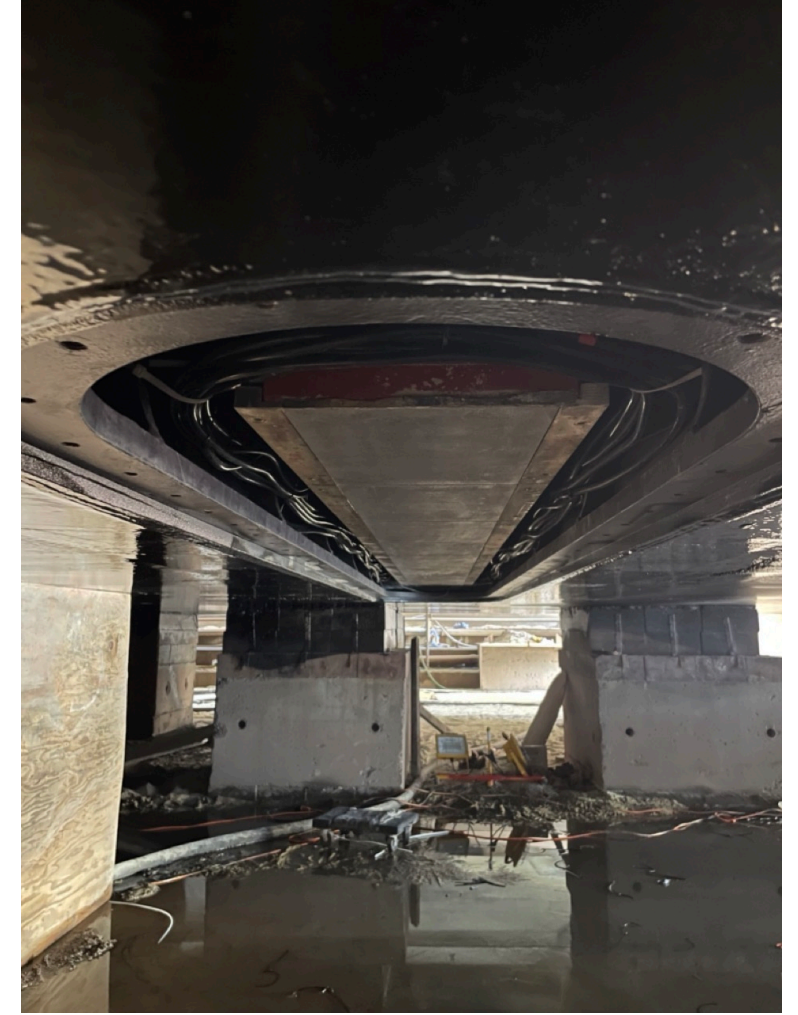
EM122 RX Array Installed
