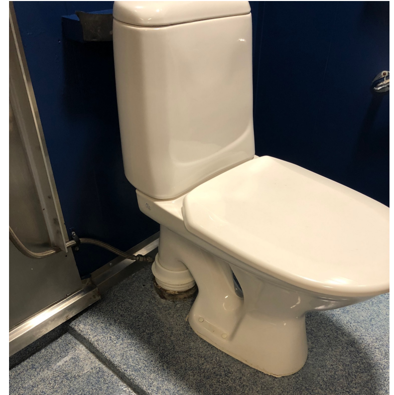
New installed heads on R/V Langseth sourced in Europe due to the flange and piping size.
