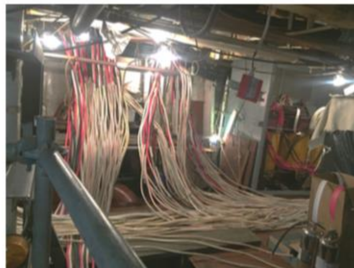
Cables prepared for feeding into switchboards
