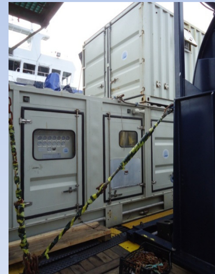
Outdoor Sarmiento's LMF® compressor
