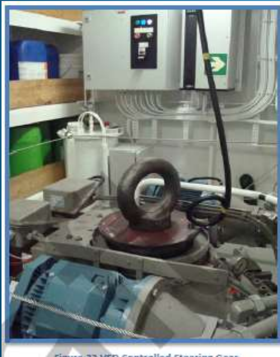
Figure 23 VFD Controlled Steering Gear
