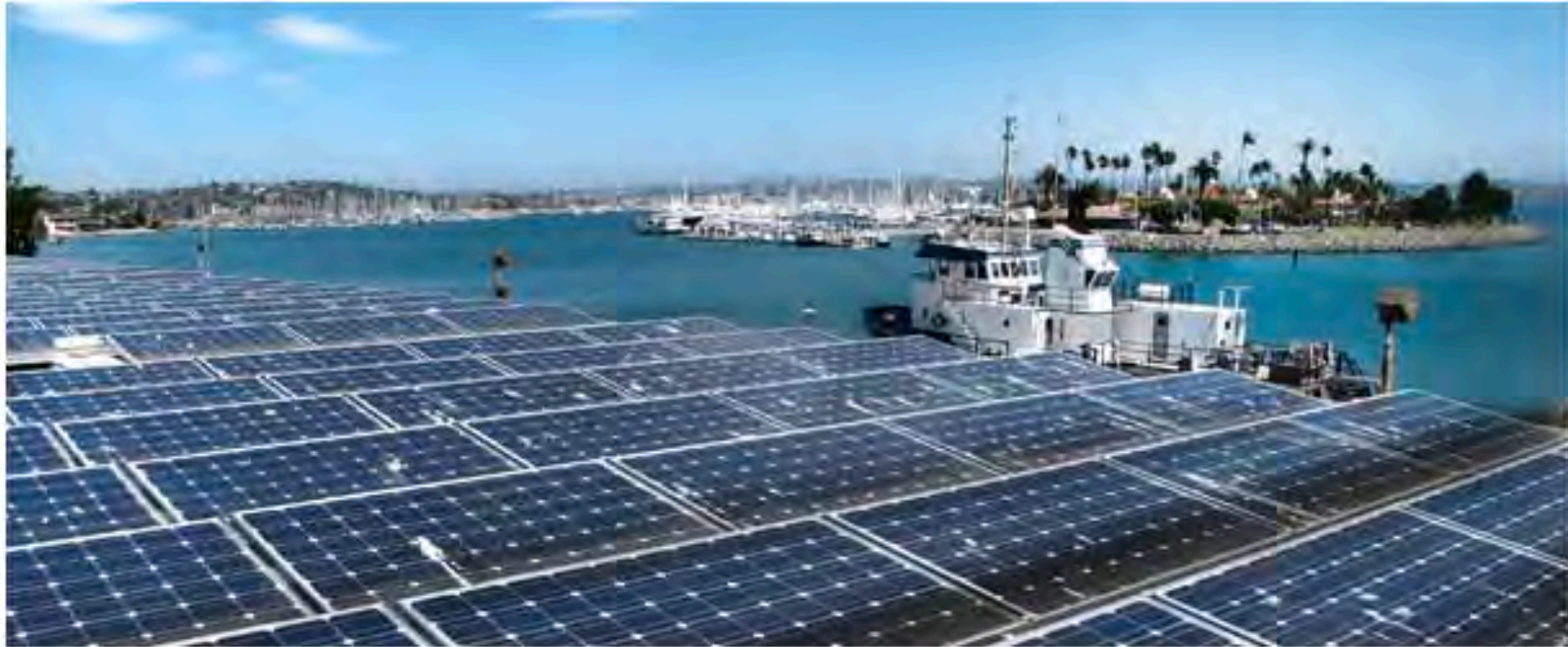
Nimitz Marine Facility installs photovoltaic system
