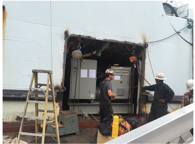
1 st seismic compressor coming out
