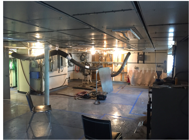
Computer Lab gutted
