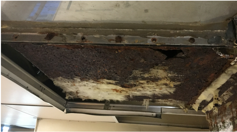
Badly corroded vent ducting
