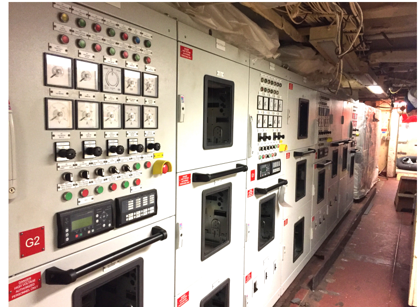
New switchboards in place
