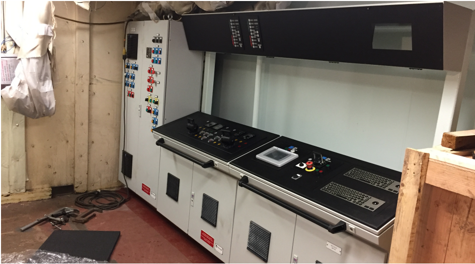
New Main Control Console in place
