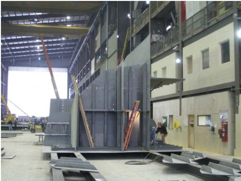
Figure 5: The start of the first module, which is just forward of the main machinery room.
