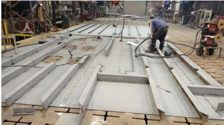
Figure 4: In preparation for starting to fabricate modules, the cut plate and shapes are joined together to form panels.
